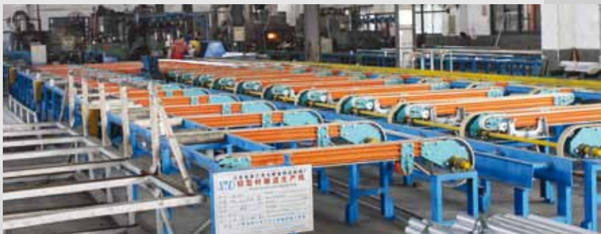
冷床 Carry-over Bed
